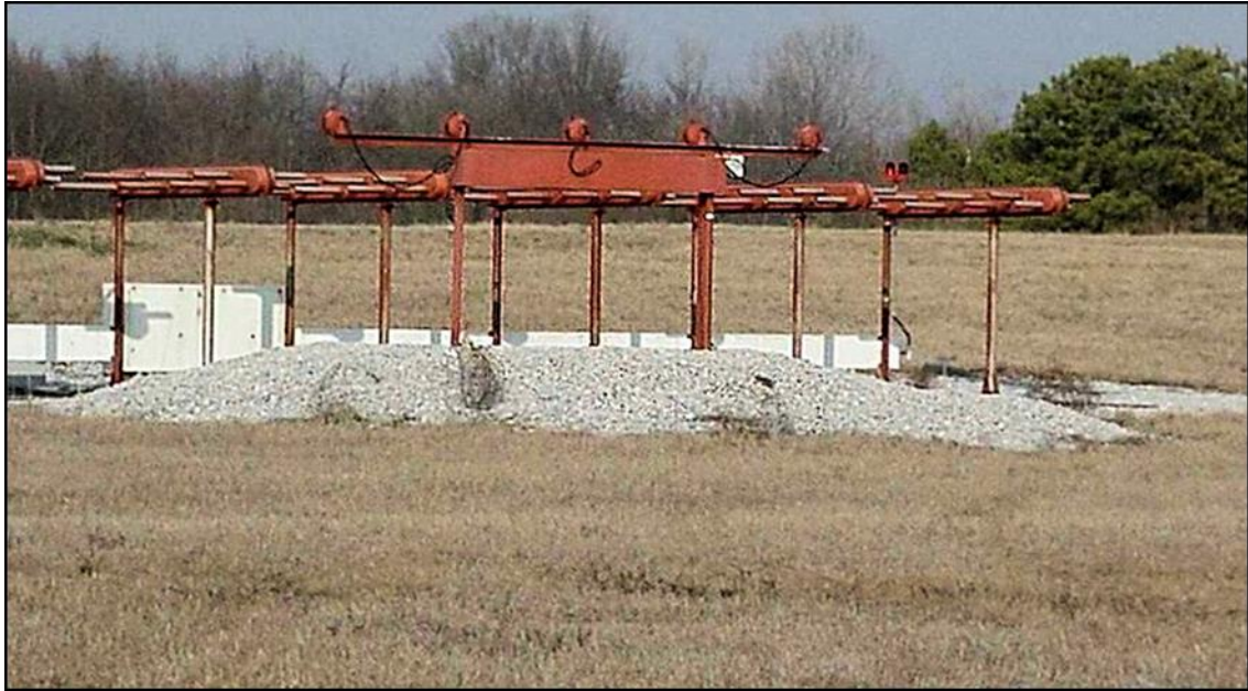
Excessive gravel fill creates a hazard
