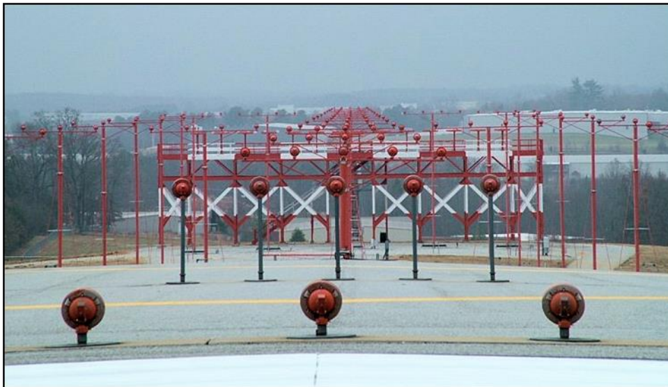
Standard ALS installation. Note electrical metallic tubing (EMT) with frangible couplings installed on light stations that are less than 6 feet high.
