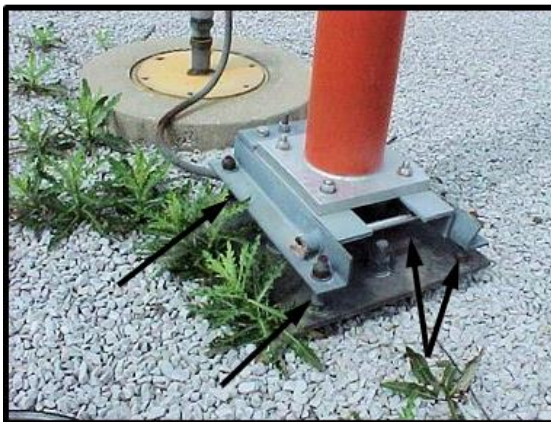
LIR structure - needs frangible bolts
